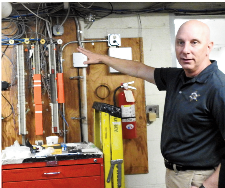
Jackson County Sheriff Gary Schuette points out a panel that powers the downtown jail's phone and security services. The panel is mounted below pipes that regularly leak water and sewage.
